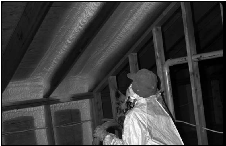
Figure 3. The specifications for most spray polyurethane foams include maximum thickness limitations. To obtain approval for thicker foam installations, a manufacturer must conduct full-scale testing of the foam's flame-spread and smoke characteristics. [Photo credit: BASF Polyurethane Foam Enterprises]
